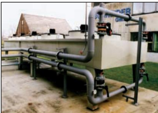
Figure 10. The dry cooler installed in the system [16]
